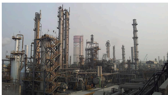
Fig. 4. The Phulpur ammonia factory in Allahabad, India. Photo from Casale SA. The size of the full industrial complex is around 800 m by 800 m.
